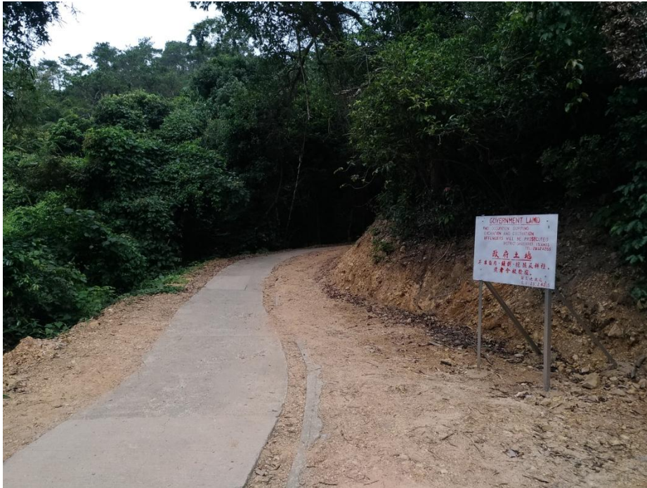
Figure 1-2 Road widening, slope cutting works and vegetation clearance were once spotted along Tung O Ancient Trail and caused adverse impact on the landscape character in the Plan Area
